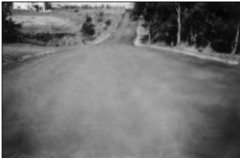
This high traffic road uses recycled asphalt place on a gravel bed.
