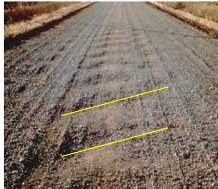
This type of washboarding appears at an angle across the roadway with ridges and depressions two to three feet apart. It is caused by excess grader speed.
