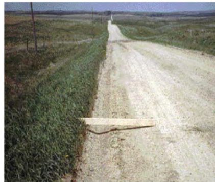
Secondary ditch over six inches deep.
